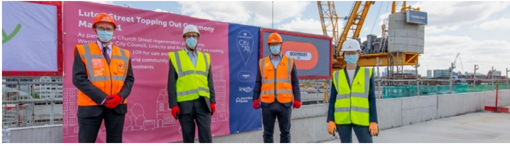
Rob Bradley (CEO Bouygues UK), Axel Boutrolle (Managing Director Linkcity), Augustin Du Four (Luton Street Project Director Bouygues UK) and Cllr Rachel Robathan at the Luton Street Topping Out Ceremony
